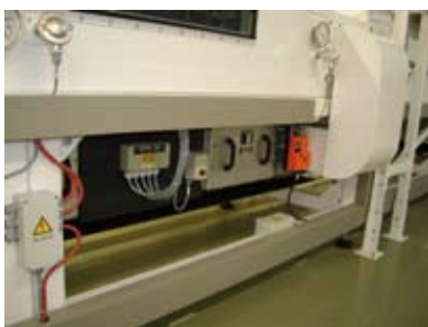
el. heating unit for the drying section
